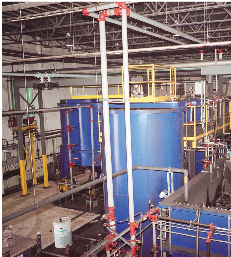
The complexity of a good system - tanks, pipes, water flow, pumps - a very comprehensive overview of an industrial wastewater treatment system.
