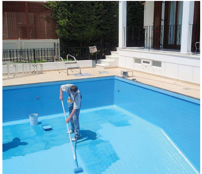
Epoxies offer a reliable, waterproof inner lining for swimming pools.
