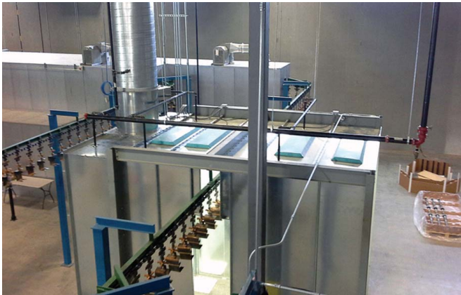
An Annadale Finishing Systems spray booth.
