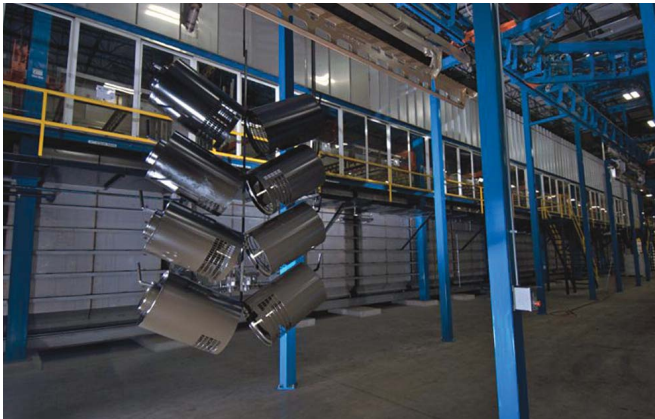
A TTX SST conveying system.
