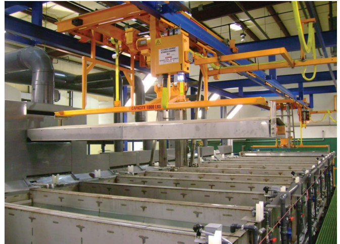
A Jessup Engineering plating system with a 1000-lb hoist.
