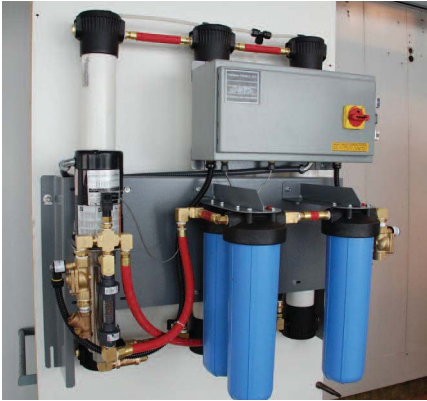
TTX Environmental reverse osmosis unit.
