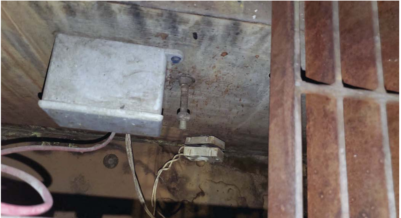
Water bug installed in the pit to shut off water to the building if it gets wet.
