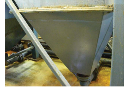
The "conical bottom" of a clarifier showing how the sludge is confined (concentrated).
