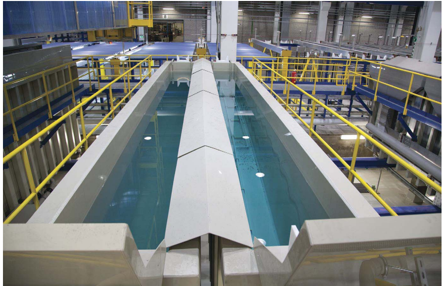
Galvatek aluminum plant with cascade rinse steps which saves water usage and improves rinsing result.
