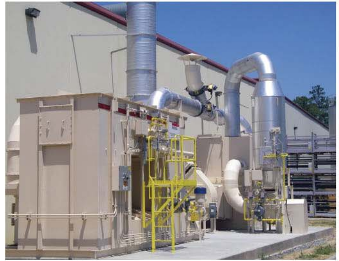
When coupled with a concentrator, oxidizers can operate with very little additional natural gas consumption due to the rich stream of emissions.
