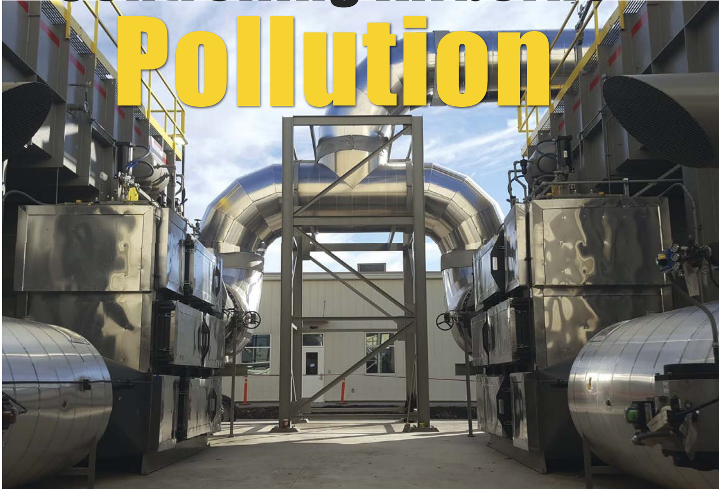
Two side-by-side Anguil model 200 Regenerative Thermal Oxidizers installed at a California facility.
