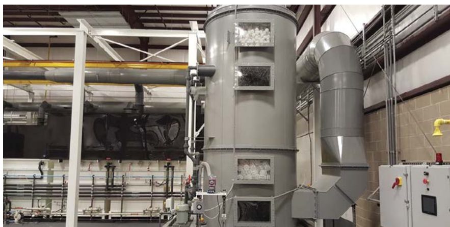
A vertical scrubber from Mech-Chem.
