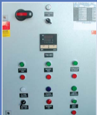
Electrical Control Panel
