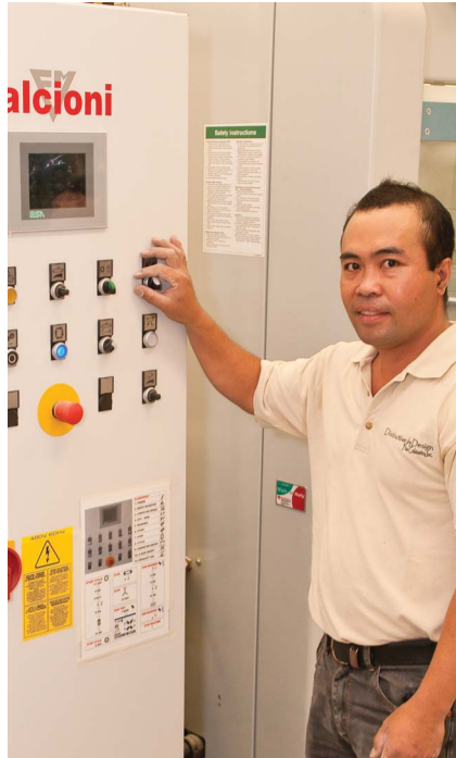
Rosendo inspects the Cefla/Falcioni; control cabinet of model Kleenspray 12.
