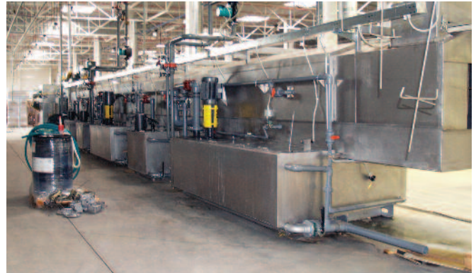
An anodizing line installed by Amiberica.
