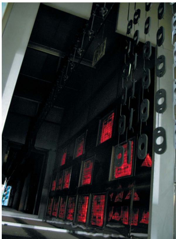
At Soucy Group in Drummondville, QC, the final cure is done using a polymerization oven with a Sunkiss Thermoreactor, which uses infrared to heat and polymerize the powder. The IR technology reduces curing time by as much as 50 per cent compared to standard convection ovens. At a line speed of 5 fpm, parts spend 18 minutes in the curing oven. At 2 fpm, parts spend close to 45 minutes in the curing oven. Cooling time is also reduced because the IR technology heats only the surface of the part. Parts under half an inch thick typically cool in 20 minutes while thicker parts take up to 50 minutes to cool. Photo by Réjean Morin of Soucy
